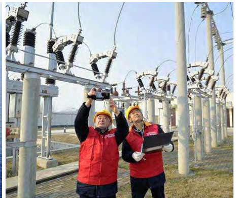
STATE GRID Zhejiang Hangzhou Branch
